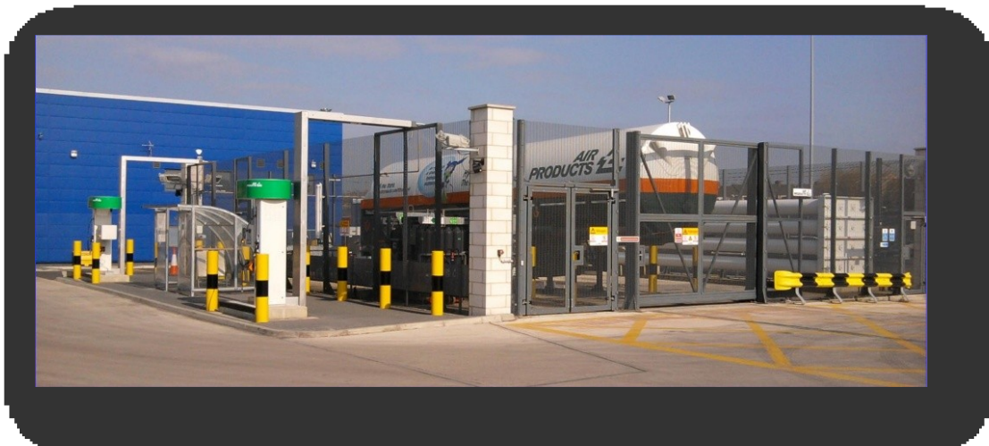
SmartFuel® fueling station at Transport for London, featuring the Air Products Dual Phase hydrogen tanker and serving a fleet of 8 fuel cell buses.
