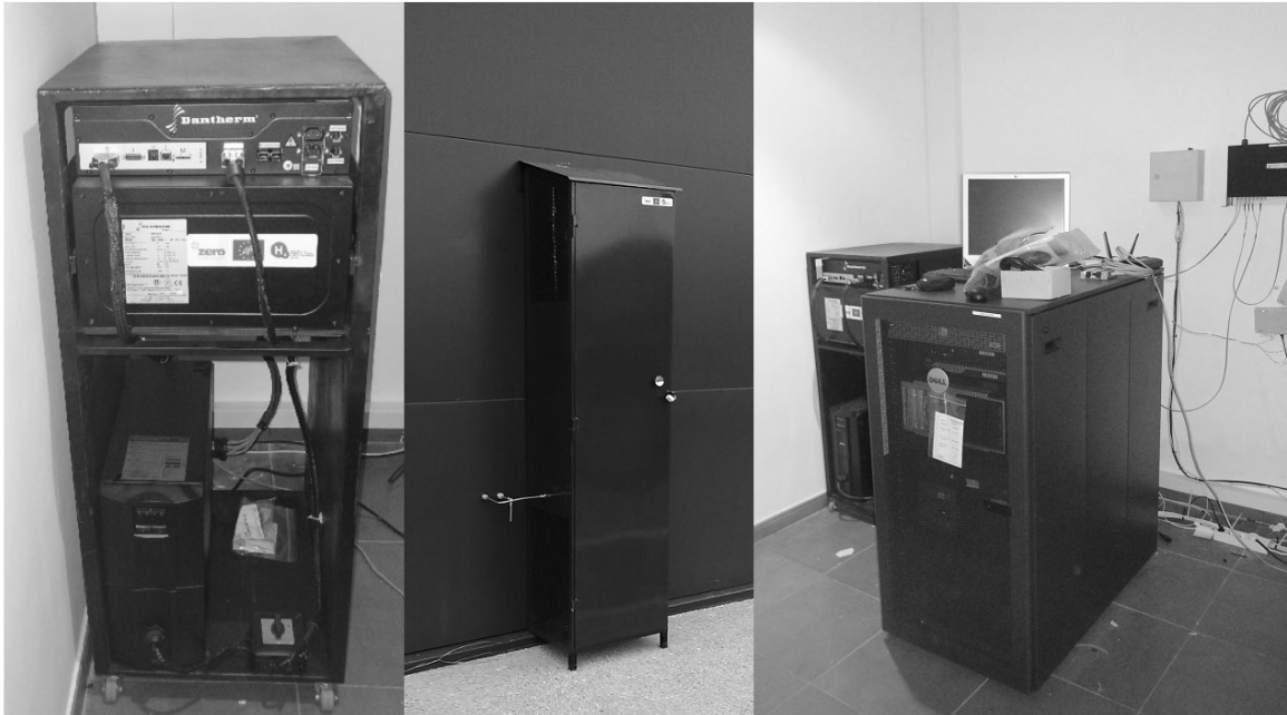
Illustration 1: Backup system, hydrogen storage and overall view with central server
